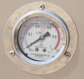
Pressure before pump out
